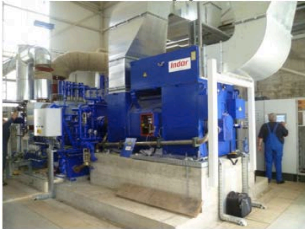
Set turbine i agregata
