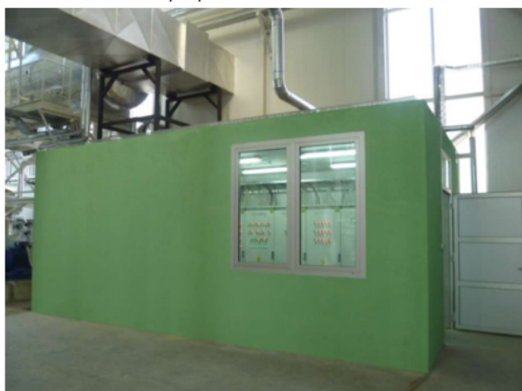
Electrical equipment for boiler control
