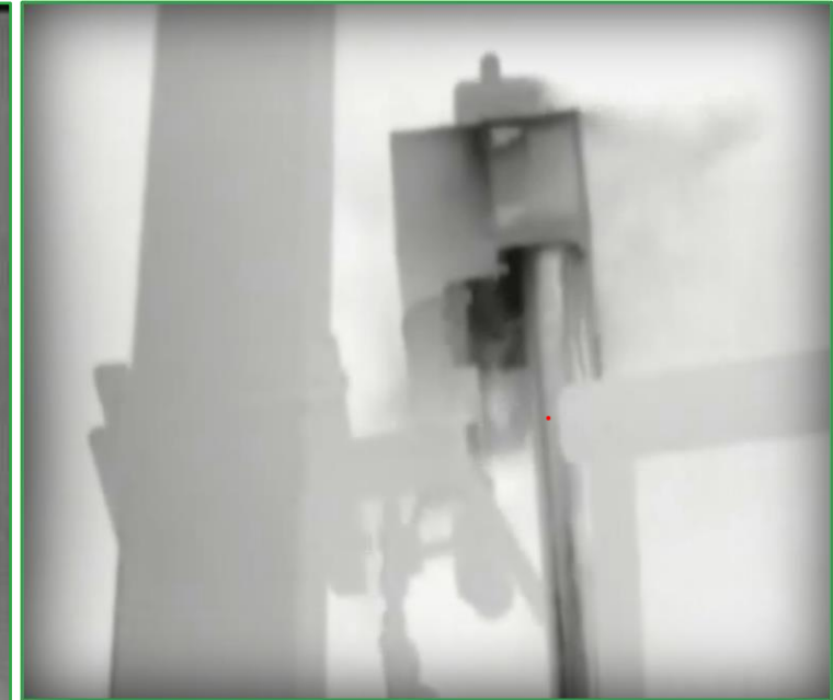
Leaking Sulfur Hexafluoride SF6 GF306 – Low Resolution
