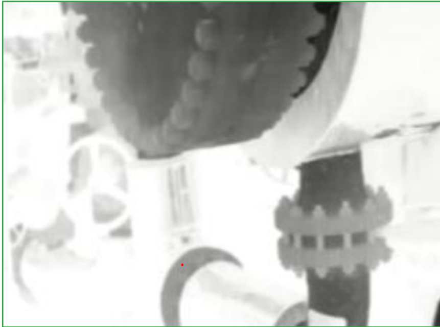
Leaking Flange GF320 – Low Resolution
