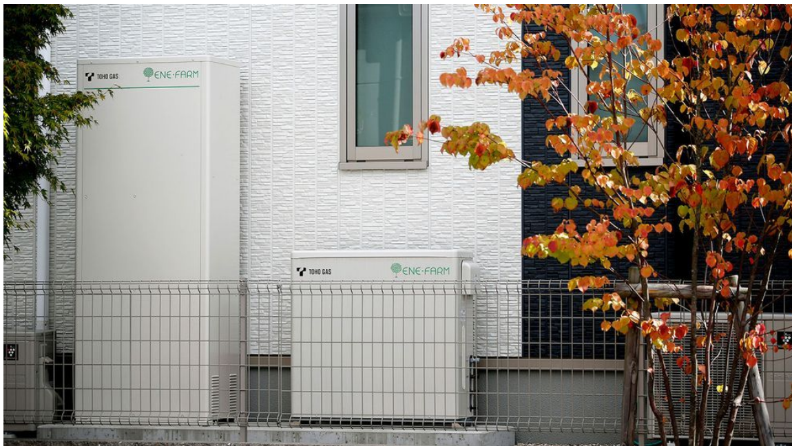
Figure 21 An example of a domestic Ene-Farm CHP unit in-situ
