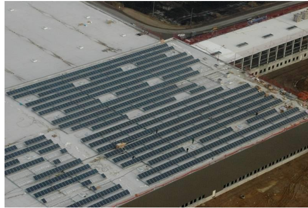
Solar (PV) Power Plant
