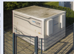
Central electricity storage
