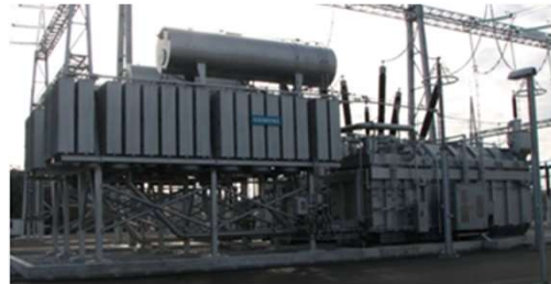
PST Phase shifting transformer
