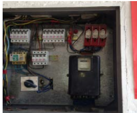
Figure 6: old distribution board
