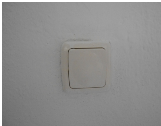
Figure 6: New manual switch
