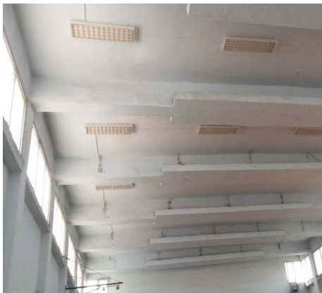
Figure 5: New surface mounted luminaries
