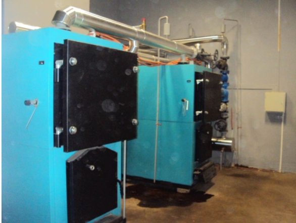
Figure 3: Energy efficient boilers
