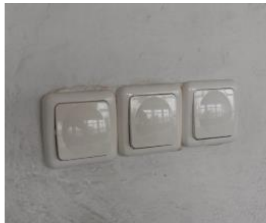
Figure 6: New manual switches
