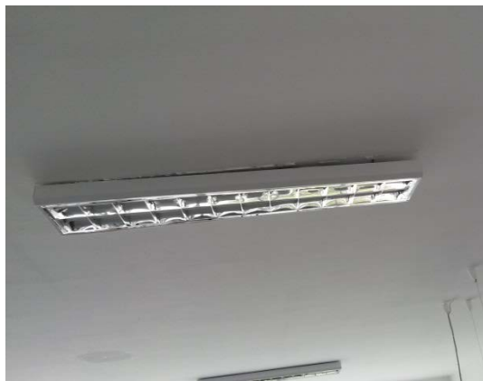
Figure 5: New surface mounted luminaries
