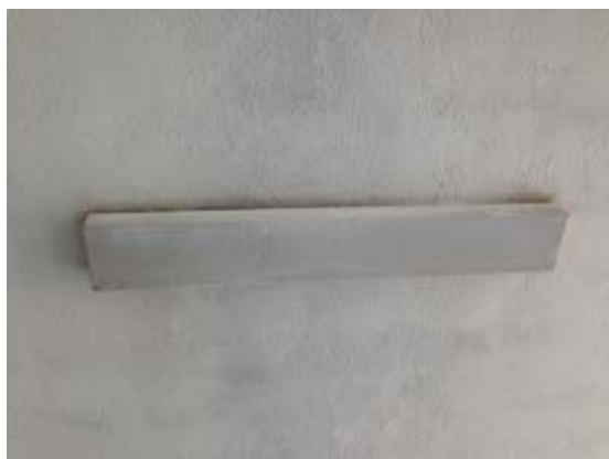
Figure 5. surface mounted luminaries
