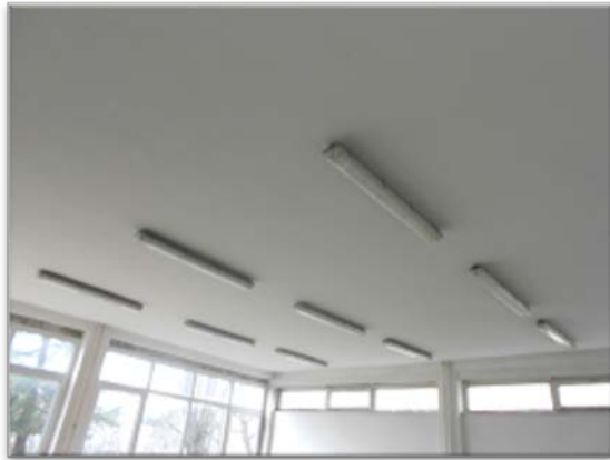
Figure 5: Surface mounted luminaries
