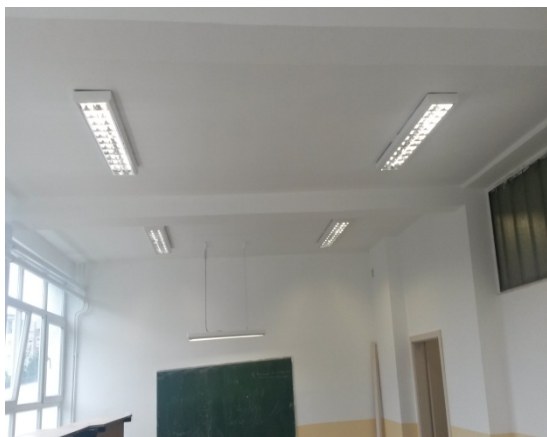
Figure 5: New surface mounted luminaries
