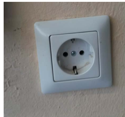
Figure 6: New electrical socket
