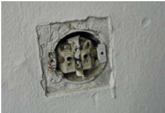
Figure 5: old manual switch
