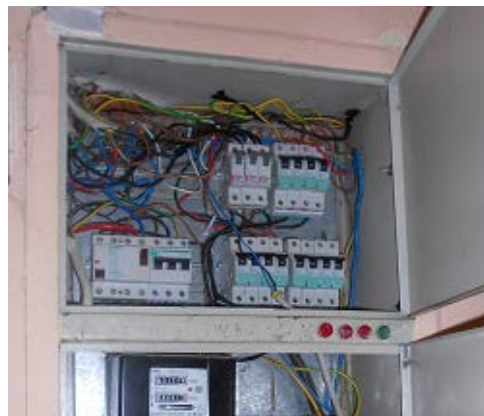
Figure 6: old distribution board
