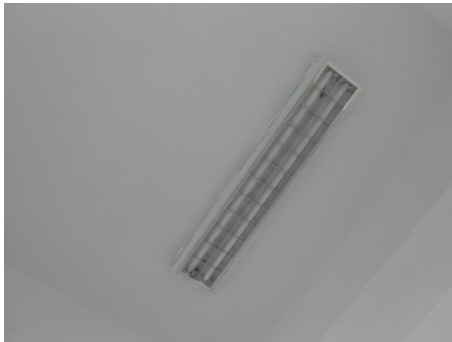
Figure 5: New surface mounted luminaries
