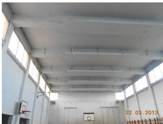
Figure 5: Surface mounted luminaries
