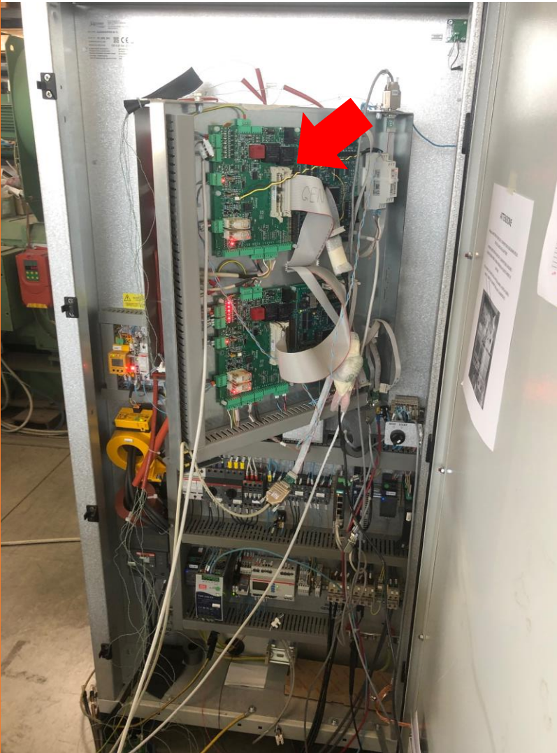
INVERTER PANEL control board
