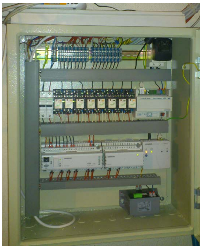
Picture 1. DDC controller with supplementary elements for regulation of the system for radiator heating and fan coils heating in the building
