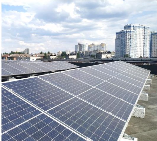
30 kW photovoltaic system
