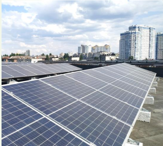
30 kW photovoltaic system
