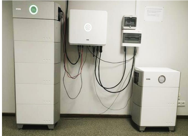
25 kWh energy storage system
