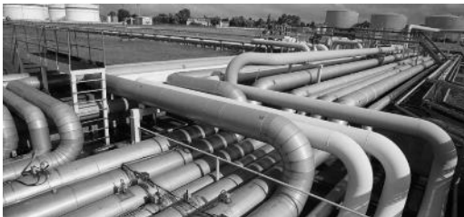
State fuel reserves terminal
