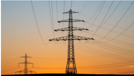
ELECTRICITY SUPPLY FROM THE GRID (TRADING)
