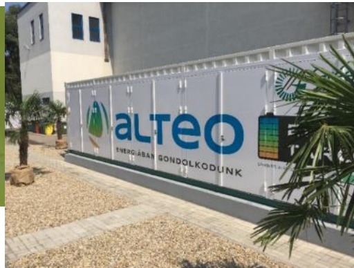
Battery electricity storage facility (from outside...)
