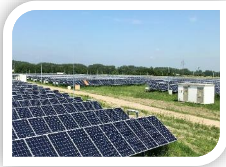
Solar power plant
